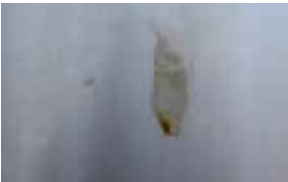
A scrubbing rinse with water does not remove these traces. The stainless steel is corroded.
