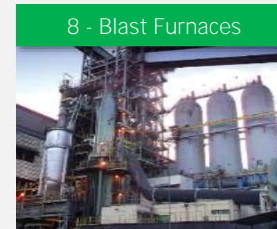
Green steel production with Aperam's BF's using renewable zero emission charcoal as a thermo-reducer
