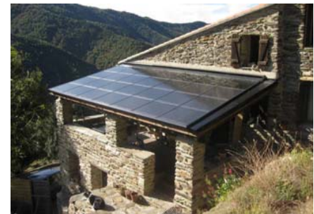
PV Solar systems
